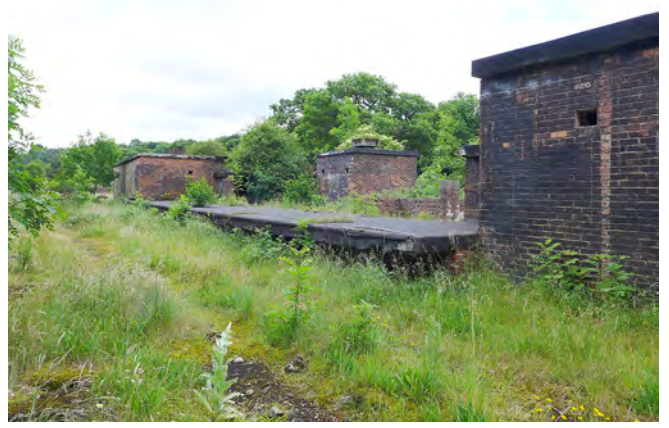
The ‘goods in’ railway loading dock in the ‘Danger Area’ at the south end of the site. The dock is coated with Colas to reduce the risk of sparks
